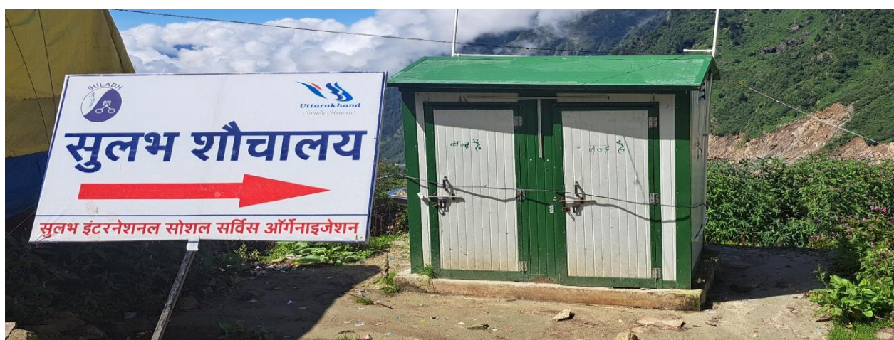
Photo 4. Locked toilets due to the filling up of sewage pits have led to reversion to open defecation in some places
